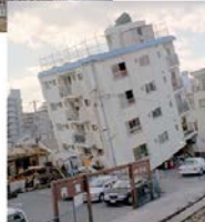
1 st floor collapse of a RC building
