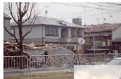
Collapsed Wooden house
